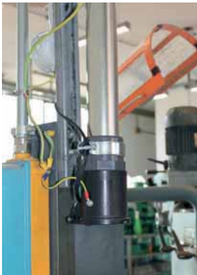
External industrial inlets
