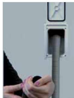
3 – lightly cover the entry: the hose will be "sucked down" in the pipe network
